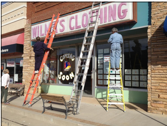
Volunteers worked on the new storefront library. More than 4,500 hours were volunteered to make the library a success.
